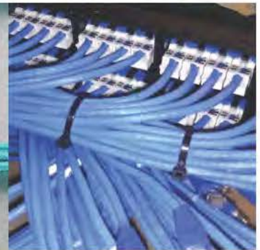
Ethernet & "Rack and Stack" Servers
